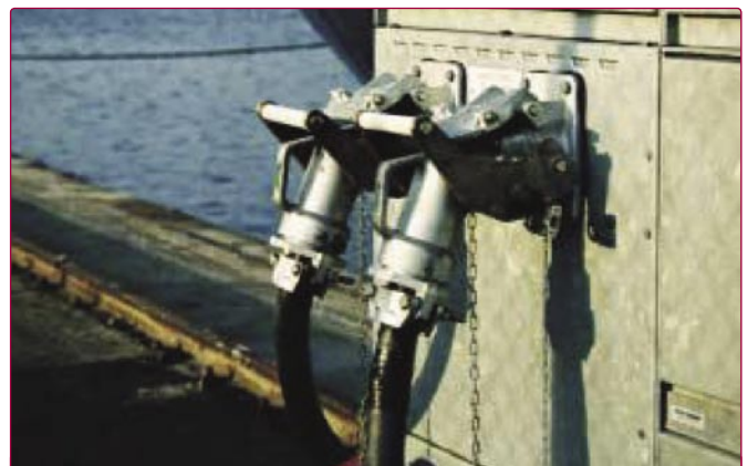
Figure 3. Shoreside electrical plugs.
